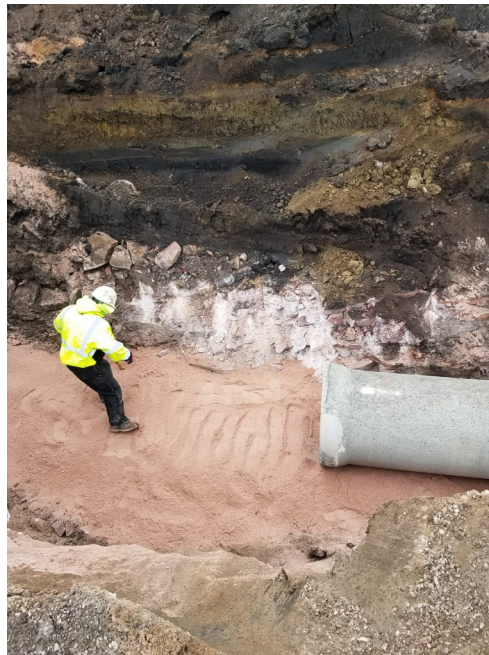
Installation of the storm sewer pipe. Bedrock is only a few feet below ground requiring blasting and rock excavation for the installation of the water main and storm sewer on the project.
