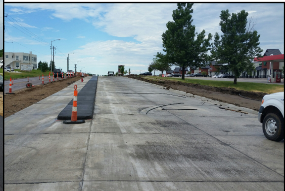
69th Street, looking west near the 69th Street and Western Avenue intersection, with concrete pavement and the median complete.
