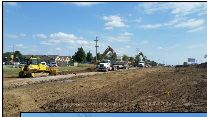
Western Avenue, looking south near the 69th Street and Western Avenue intersection, as excavators tear out the existing pavement and load onto trucks to be hauled off site.
