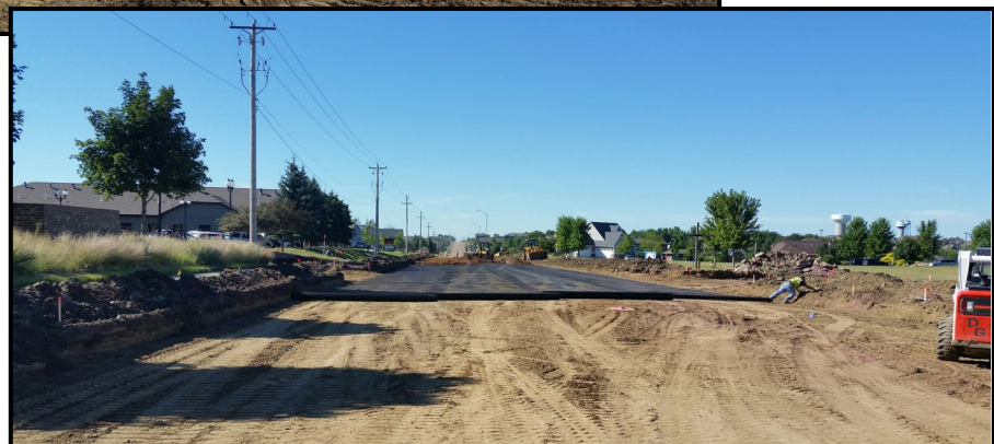
Western Avenue, looking south, near the south end of the project. Grading for the roadway is completed and geogrid is being placed along with the gravel base.
